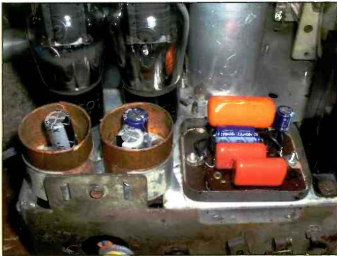
Photo C. Here's a view showing how the replacement bypass capacitors were hidden inside the original Philco capacitor bank.
